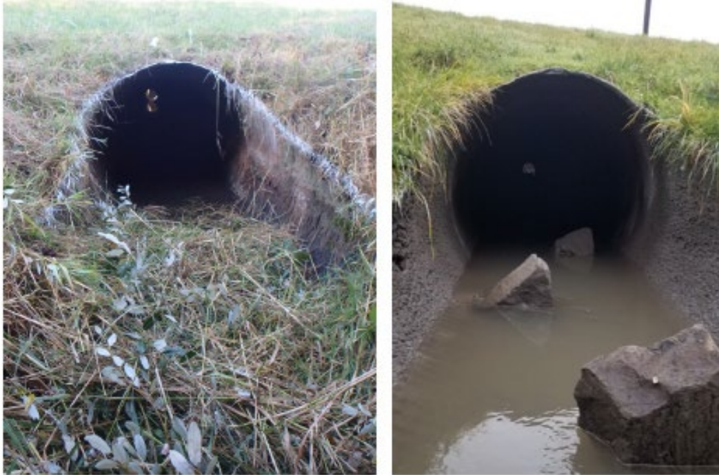
Figure 11: Unnamed Tributary to Mud Slough Culvert Repair, Before and After Description: Two images, the first is the pre-repair view inside the culvert. The second image is of fish rocks inside of the culvert post-repair with water running through it.
